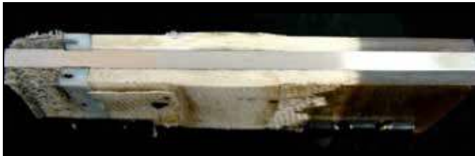
Steam attack on GRE isolation gasket
