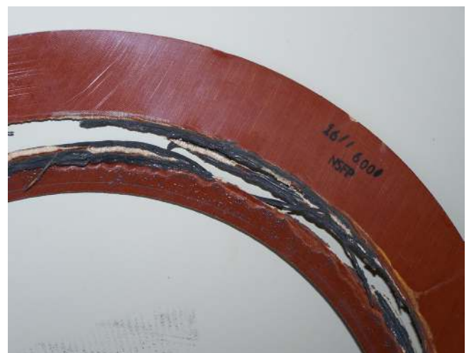
Figure 3. The tendency of phenolics to crack has eliminated them from flange isolation applications.
