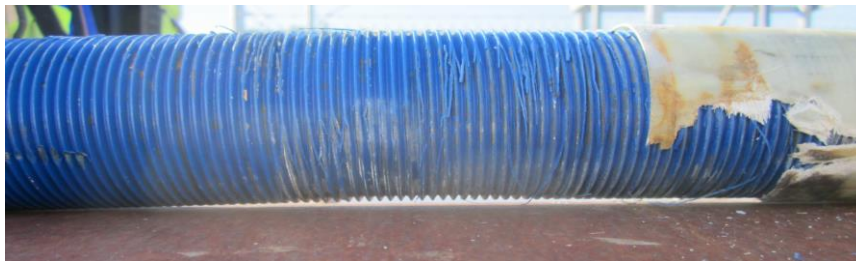
Image 3: Bolt bending due to excessive flange rotation.
