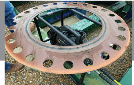
Phenolic isolation gasket removed from flange
