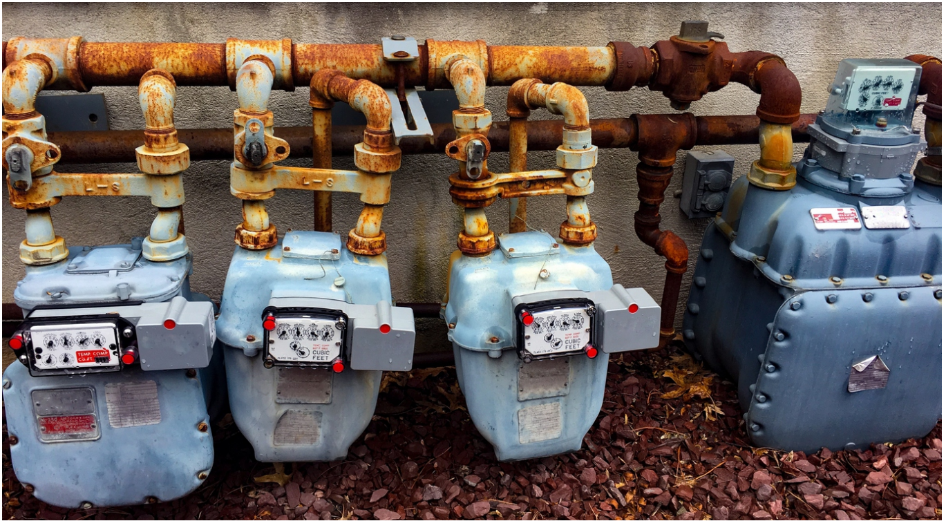
Figure 5: Natural gas meters and old rusty pipes Source: iStock
