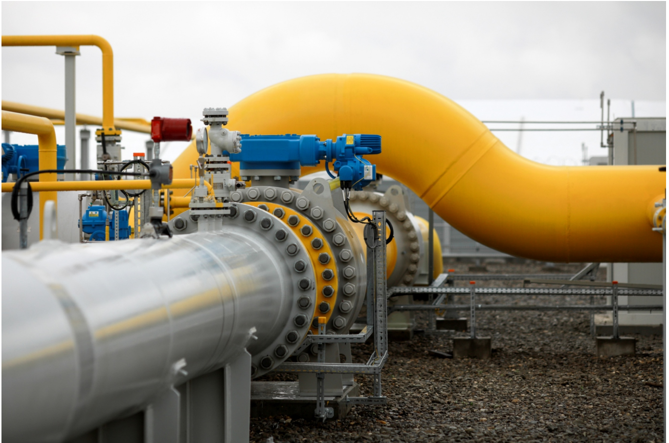
Figure 3: Natural Gas Compressor Station
